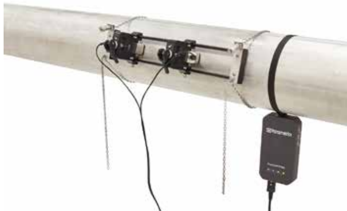
Clamping fixture, transducers and transmitter mounted on pipe
